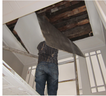
↑ Plafond removal process in Altamirano 20. March 21, 2012, 13:58 hrs. ↗ Plafond removal process in Pomona 36. May 21, 2012, 11:26 hrs.
